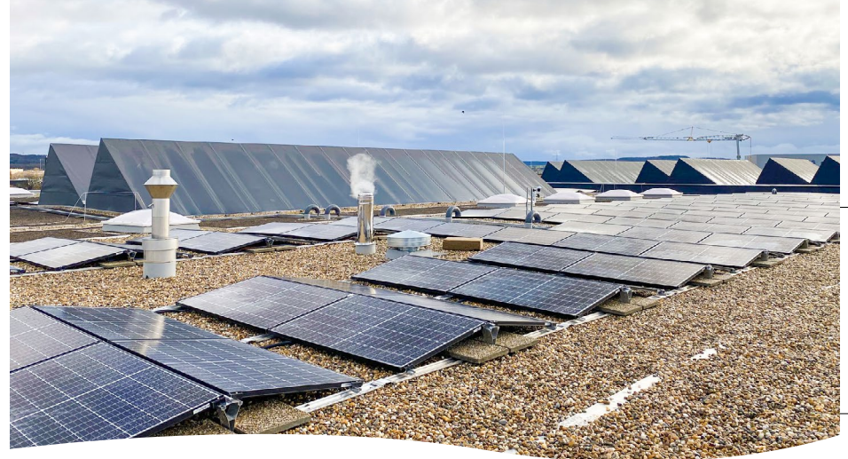
Solar panels are on part of the sustainable design of our facility in Walldorf, Germany.
